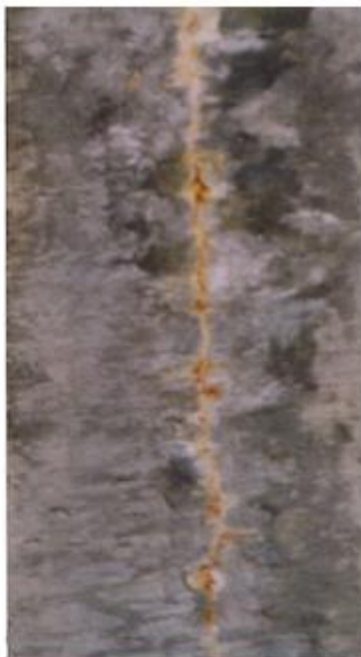
Example of deteriorated concrete pavement
